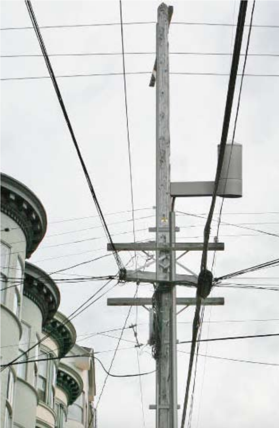
Verizon Wireless is deploying small cells on wooden utility poles in San Francisco.
